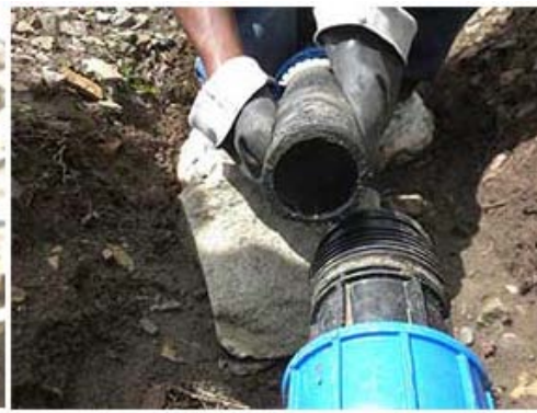
Pipe after Unacid treatment.
