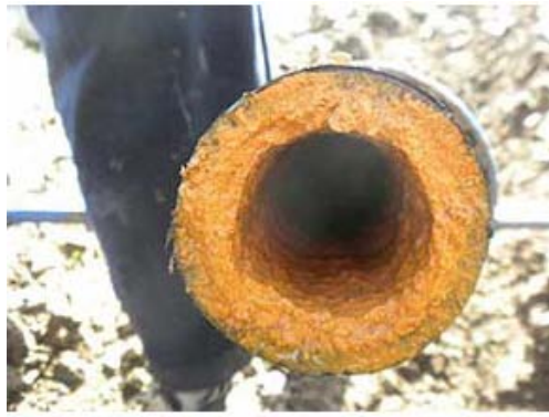
Pipe capacity at 30 meters before treatment.
